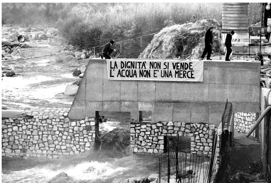
Fig. 5 – The abandoned construction site of the micro-hydroelectric plant of Mis, already partially covered with "local stone"
